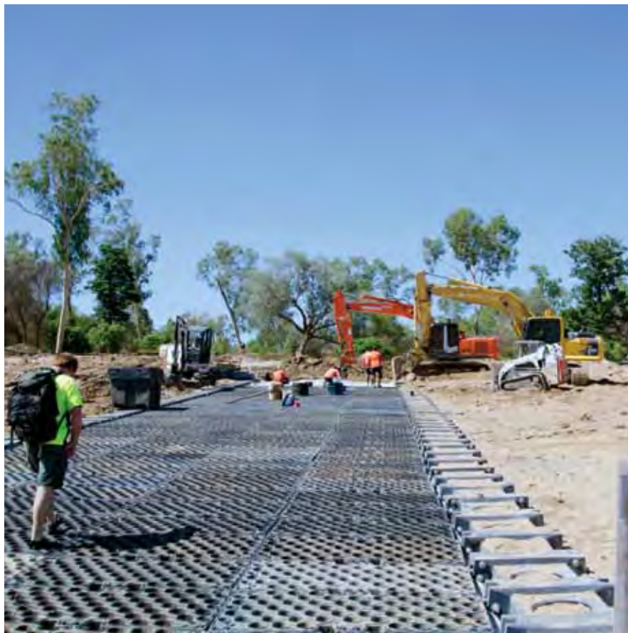
Installation of the head wall on Mitchell River crossing in North Queensland.
