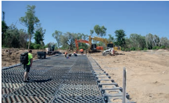
The PE structure over the Mitchell River is built during the dry season
